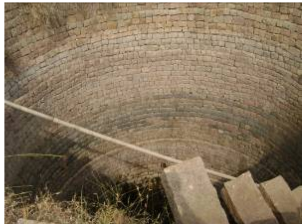
A Typical Loss of Well - needs Replacement
